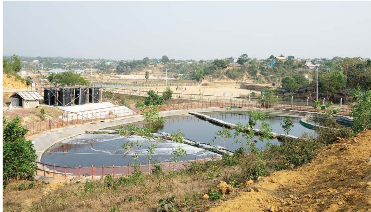
The world's largest refugee settlement, Kutupalong refugee camp, houses 745,000 Rohingya refugees in Cox's Bazar in Bangladesh. Providing clean water, sanitation and hygiene is a challenge. UNHCR, in partnership with OXFAM, operates the largest sewage sludge management plant in any refugee camp.
