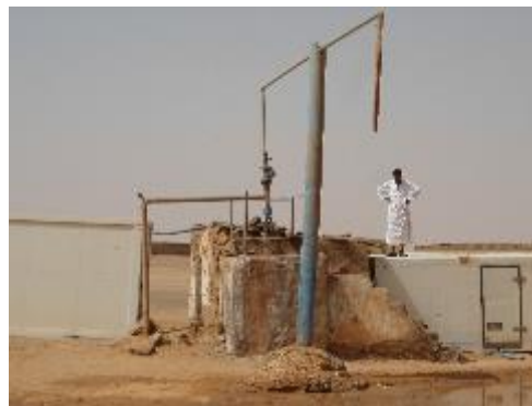
"Giraffe" system at borehole for filling water trucks. UNHCR undertook many water interventions during the hot summer months. UNHCR/M.Kachebi
