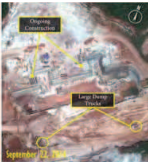
fig 3: Ongoing construction can be seen in imagery from September 22, 2014. Additional foundation footings are present along with large loaded dump trucks. The function of the large structure cannot be determined at this phase in construction.
