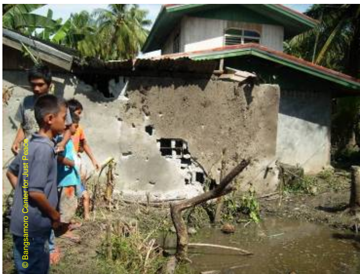
This house, close to the tents in the IDP camp in Libutan village was hit by mortar shelling
