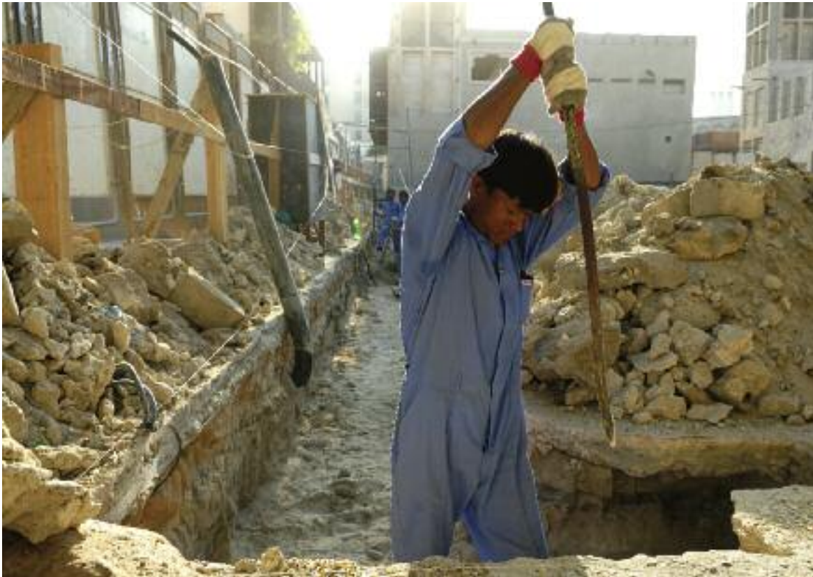
A migrant worker on a construction site in Dubai, United Arab Emirates.
