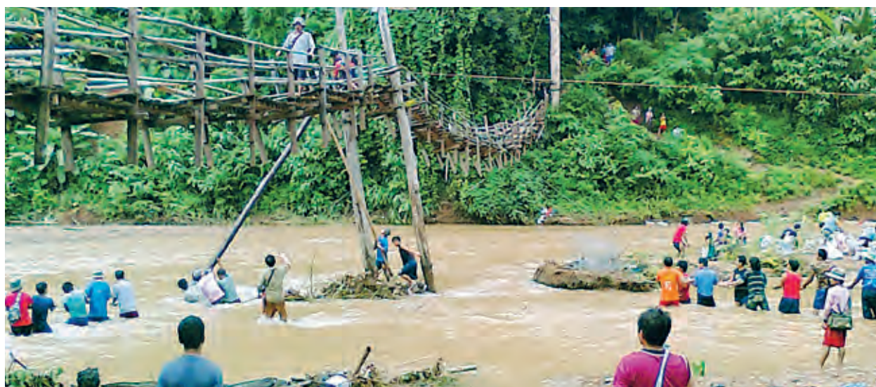
Camp residents repair a bridge in Mae Surin that was damaged by the floods.
