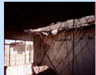
UN-HABITAT - Damaged school roof for rehabilitation
