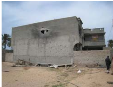
Houses hit by a Grad rocket in the Qasr Ahmad neighbourhood of Misratah, Libya, 16 April 2011. © Amnesty International
