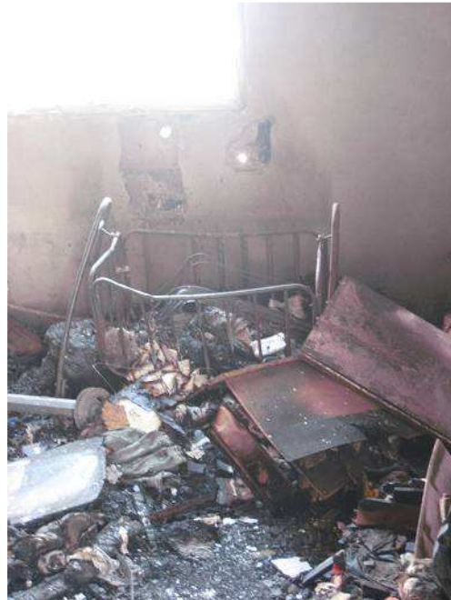
Second floor of a house destroyed by opposition forces in Benghazi © Amnesty International
