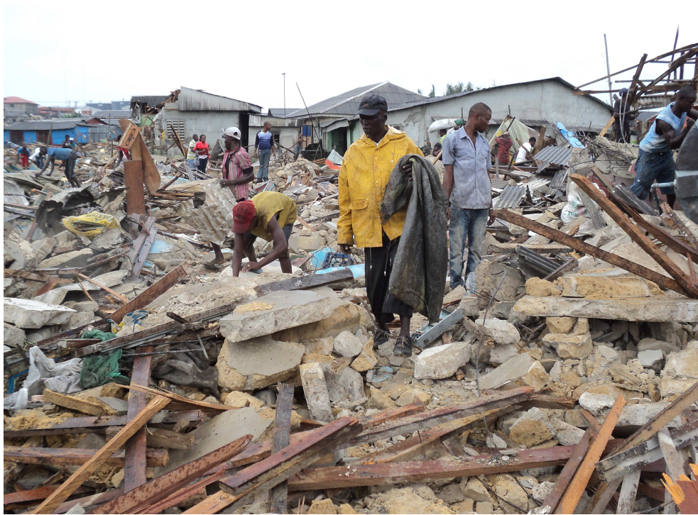
Former residents picking from the rubbles after the demolitions in Abonnema Wharf - Thursday 28 June 2012
