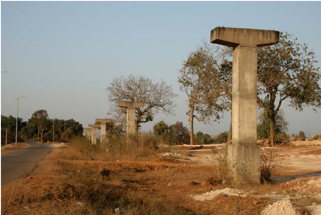
Photo 3: Pillars for the conveyor from the mine site at Niyamgiri Hills to Lanjigarh refinery (Amnesty International, taken in March 2009)
