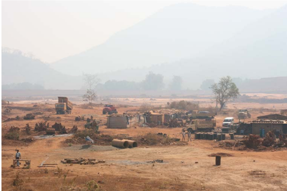
Photo 12: A view of the red mud pond under construction at Lanjigarh (Amnesty International)
