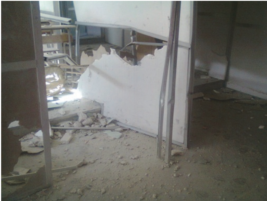
Damage caused by a mortar shell to the Akrama al Makhzoumi school. © 2013 Human Rights Watch
