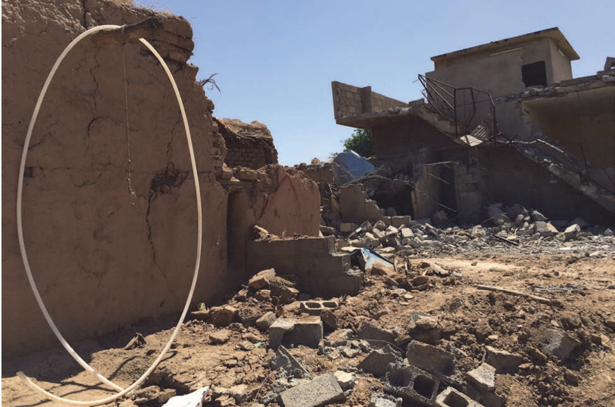
Destroyed houses in Qarah Tappah, with partial red “X” still visible, May 20, 2016. © 2016 Human Rights Watch
