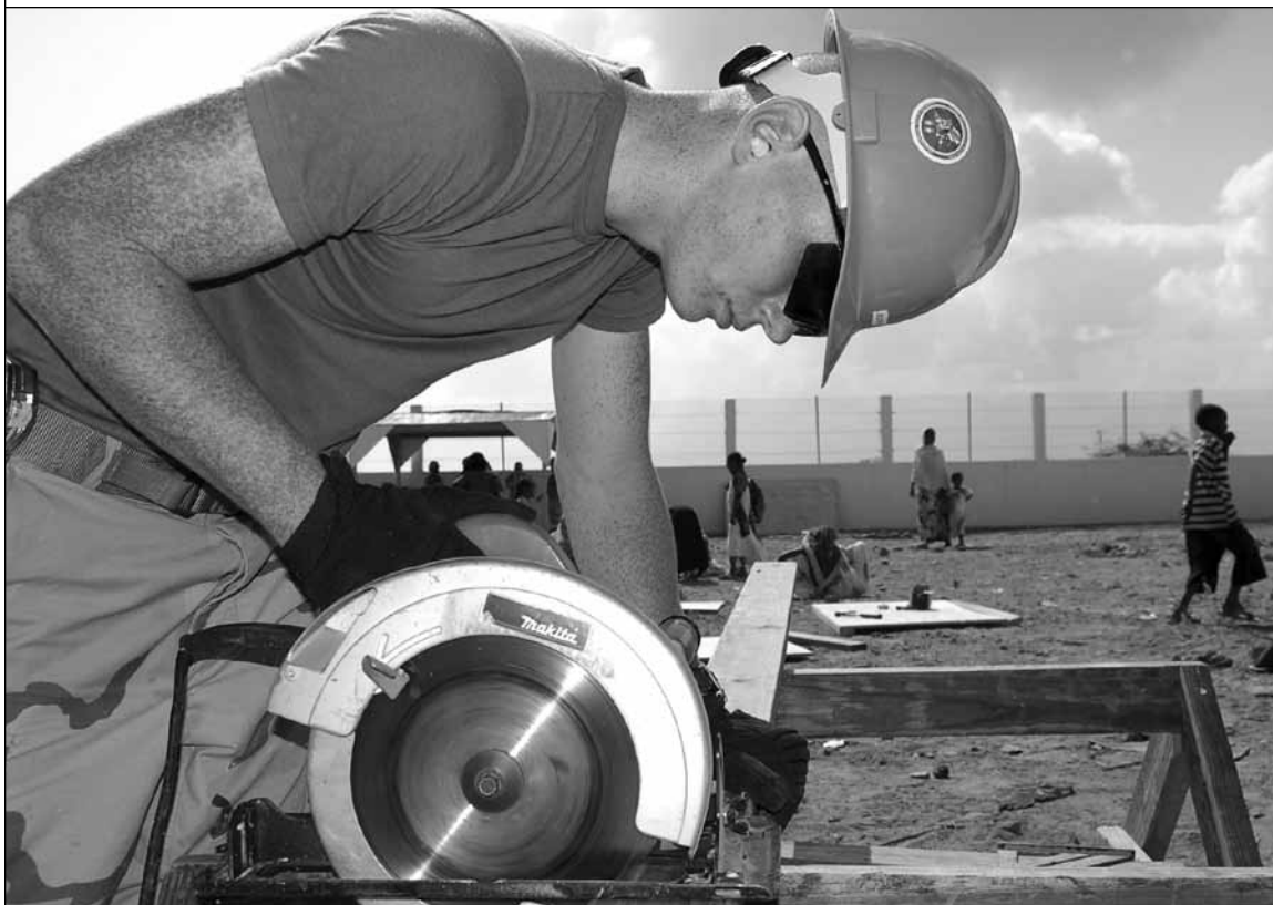
A U.S. Navy sailor cuts framework for a new primary school in Djibouti as part of a construction battalion attached to Combined Joint Task Force - Horn of Africa.
