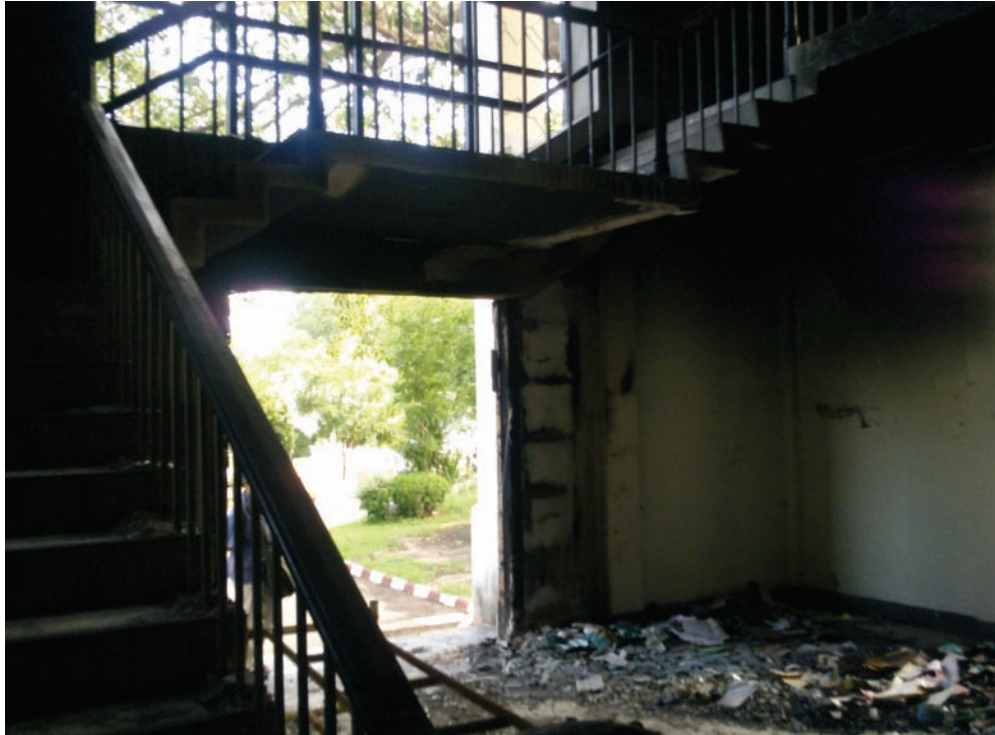
Burned-out side staircase on the ground floor of the Khon Kaen provincial hall, damaged by protesters on May 19, 2010. © 2010 Human Rights Watch
