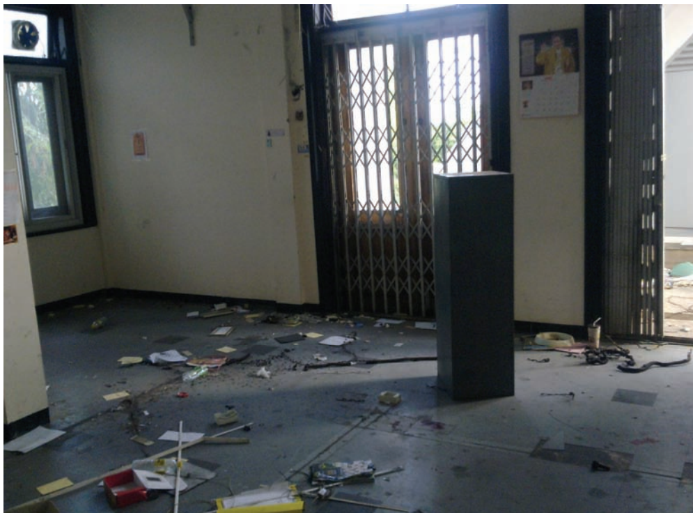
Damaged and abandoned civil service office at Khon Kaen provincial hall. © 2010 Human Rights Watch
