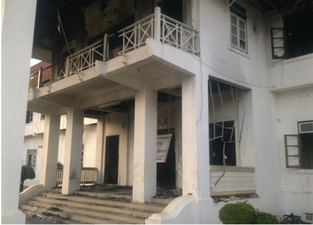
The main entrance of Udon Thani provincial hall showing fire damage after protestors burned it on May 19, 2010. © 2010 Human Rights Watch
