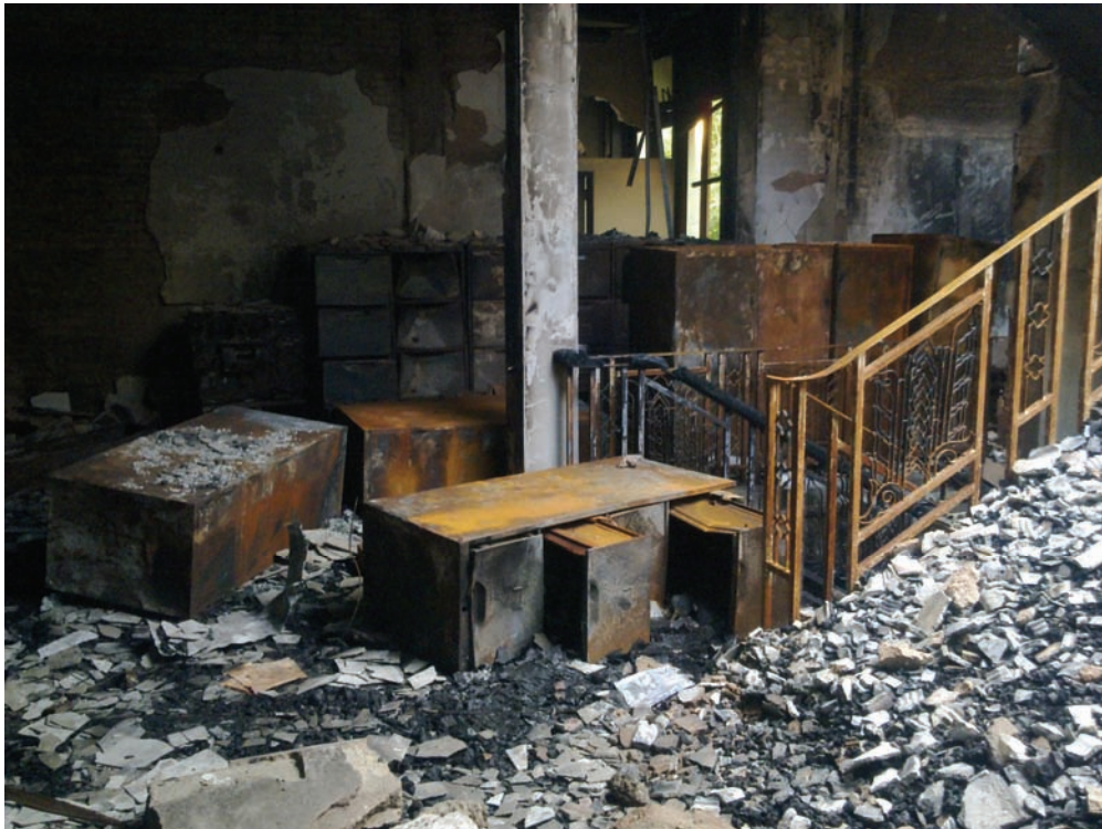
Rubble and burned-out filing cabinets on second floor of the central staircase of the old wing of the Khon Kaen provincial hall, which was set afire by protesters on May 19, 2010. © 2010 Human Rights Watch
