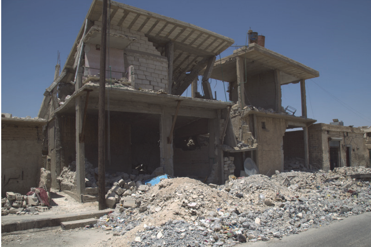
A residential house in Tabqa city that was hit by a coalition airstrike April 25 or 26, 2017, in an attack that killed 16 civilians, including nine children. © 2017 Ole Solvang/Human Rights Watch
