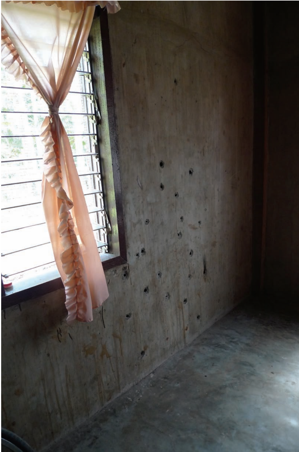
The Tambungalan family home remains riddled with holes from the bullets that killed Haji Noria Tambungalan and her child on July 20, 2005. © 2009 Human Rights Watch
