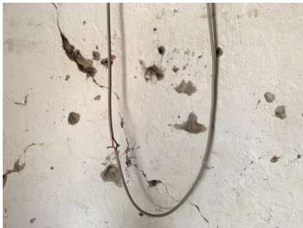
The shrapnel-scarred wall of the room in which six-year-old Joy Kamisa was killed. © Amnesty International
