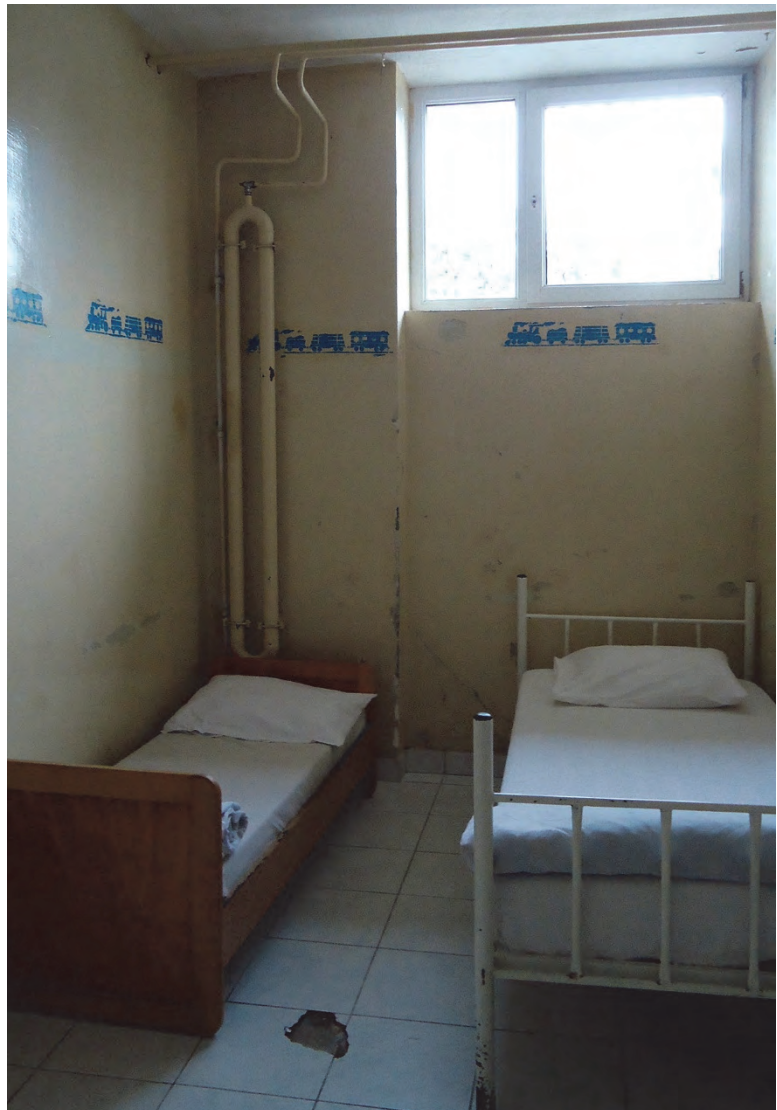
One of the isolation rooms in the Veternik institution. Isolation rooms are used to separate children and adults from other residents in cases of contagious diseases or until they “adapt” to the institution. © 2015 Emina Ćerimović for Human Rights Watch
