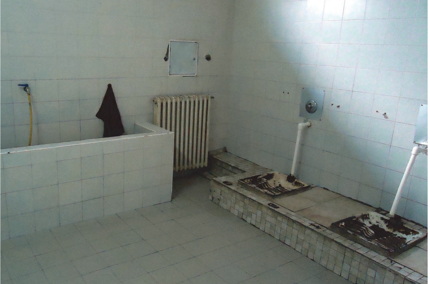
Bathroom in the Stannica Home for children and adults with disabilities. There are no doors or means of privacy separating the toilets in the bathroom. There are no showers and children use the water hose when taking a bath. © 2015 Emina Ćerimović for Human Rights Watch
