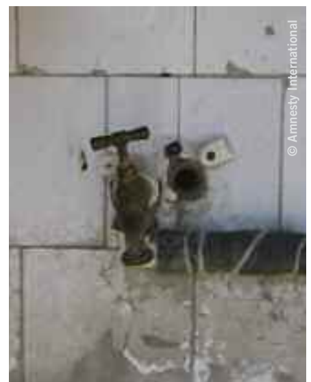
Below: The Niš authorities took over two months to connect this single tap in the warehouse that the five Romani families had been sent to.
