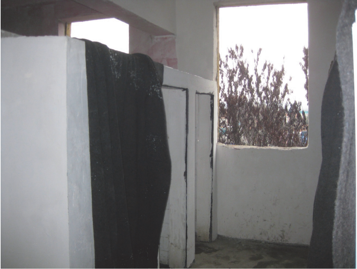
A bathroom in one of the residential buildings in Harmanli. The toilets had no doors and the windows had no glass. Temperatures were below freezing. ©2014 Human Rights Watch
