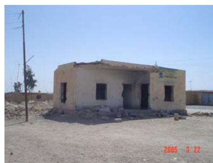
Damaged Library in Al Tash Camp - UNHCR
