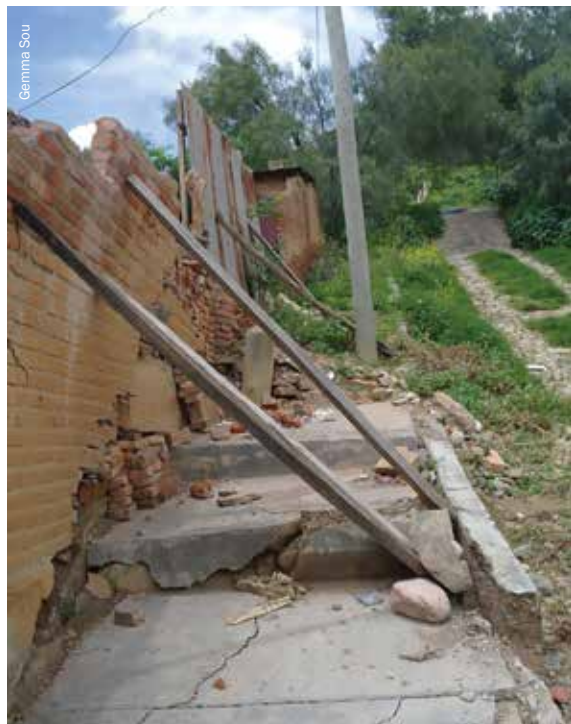
Walls propped up, post-landslide, Cochabamba.
