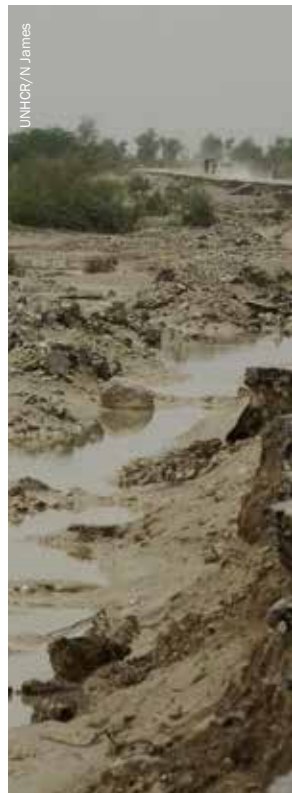
Road damaged by floods in Balochistan, Pakistan, 2010.
