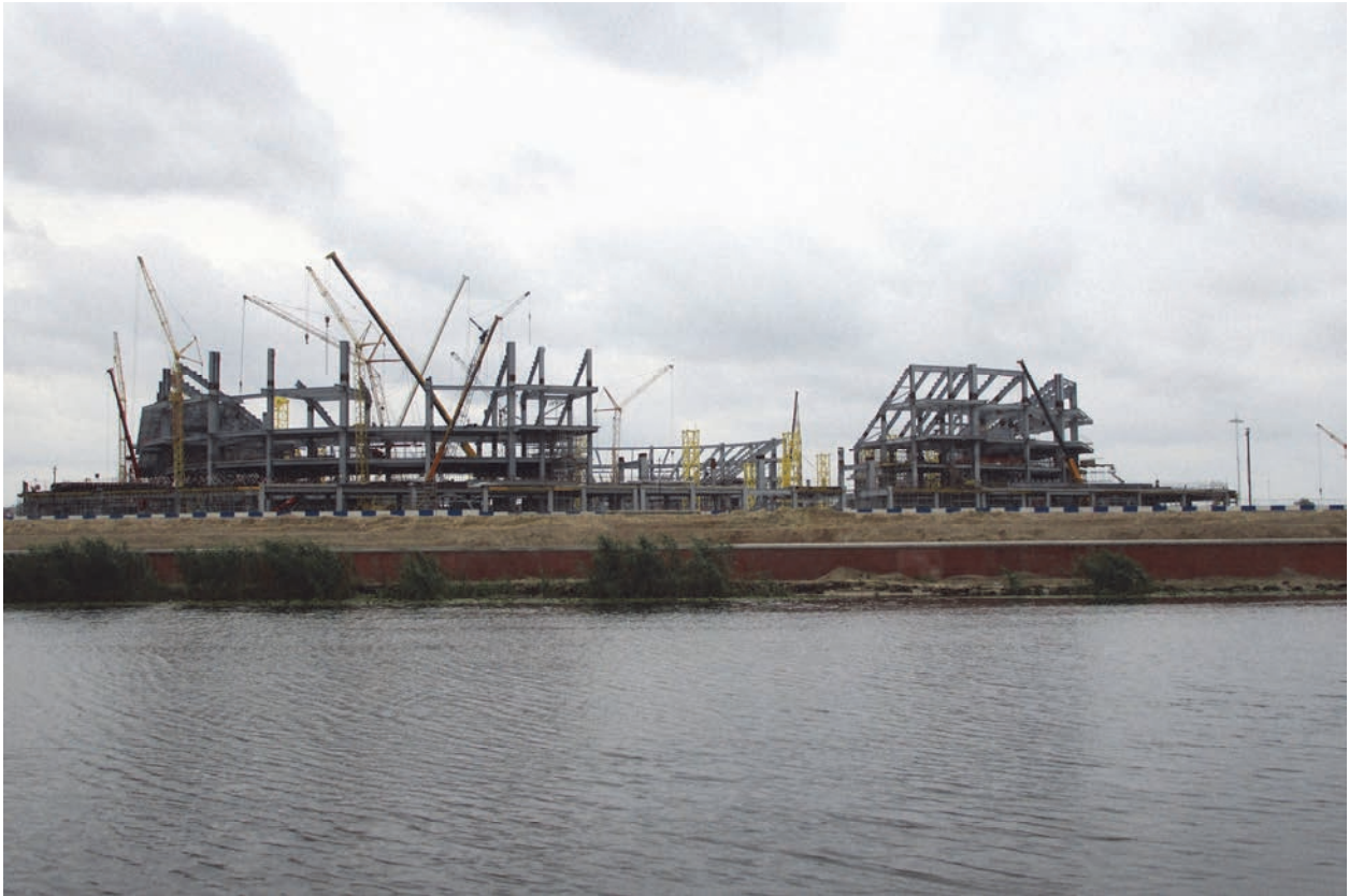
The Kaliningrad Stadium, a 2018 World Cup venue, in Kaliningrad, Russia, under construction in July 2016. © 2016 Semyon Simonov for Human Rights Watch
