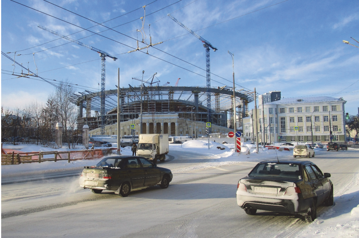
The Ekaterinburg Arena, a World Cup 2018 venue, in Ekaterinburg, Russia, under construction in January 2017. © 2017 Semyon Simonov for Human Rights Watch
