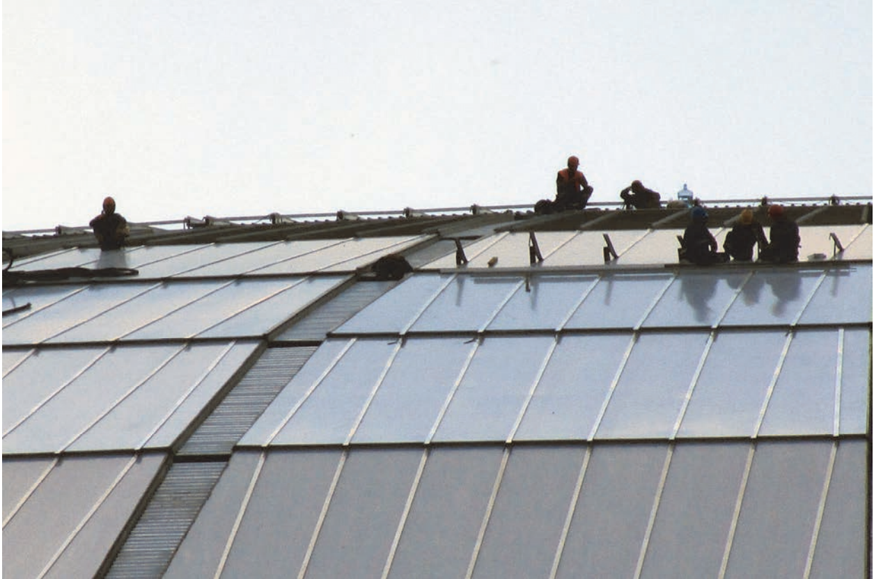
Workers on the roof of the Luzhniki Stadium, a 2018 World Cup venue, in Moscow, Russia in July 2016. © 2016 Semyon Simonov for Human Rights Watch
