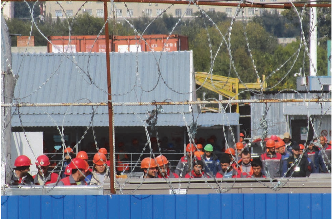
Workers on the Rostov Arena, a 2018 World Cup venue under construction in Rostov-on-Don, Russia, in September 2016. © 2016 Semyon Simonov for Human Rights Watch
