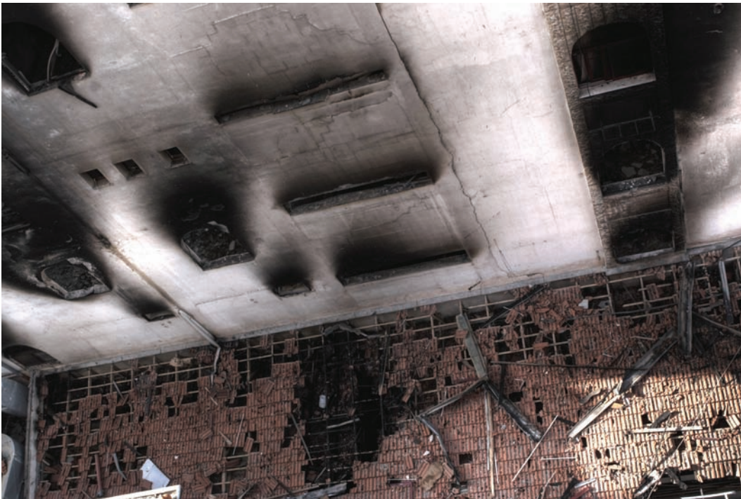
The administration building of Al-Quds hospital was gutted by fire started by white phosphorous. The hospital was hit by two white phosphorus shells on January 15, 2009, forcing the evacuation of all patients and staff. © 2009 Marc Garlasco/Human Rights Watch
