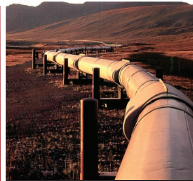
Trans-Sahara Gas Pipeline
