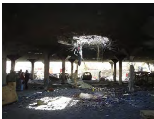
Figure 49.D.3 Post blast interior
