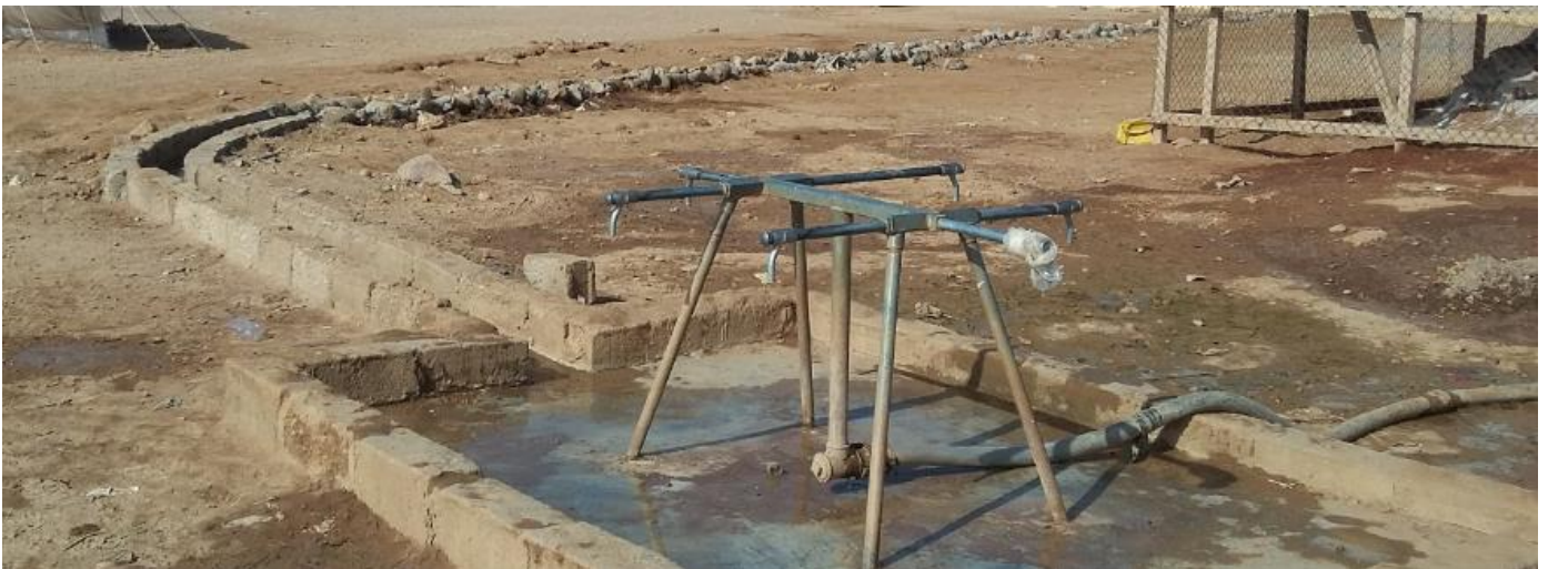
NRC has cleaned the water points in Markazi camp and constructed water trenches around them to contain and drain excess water. ©NRC/March 2016.
