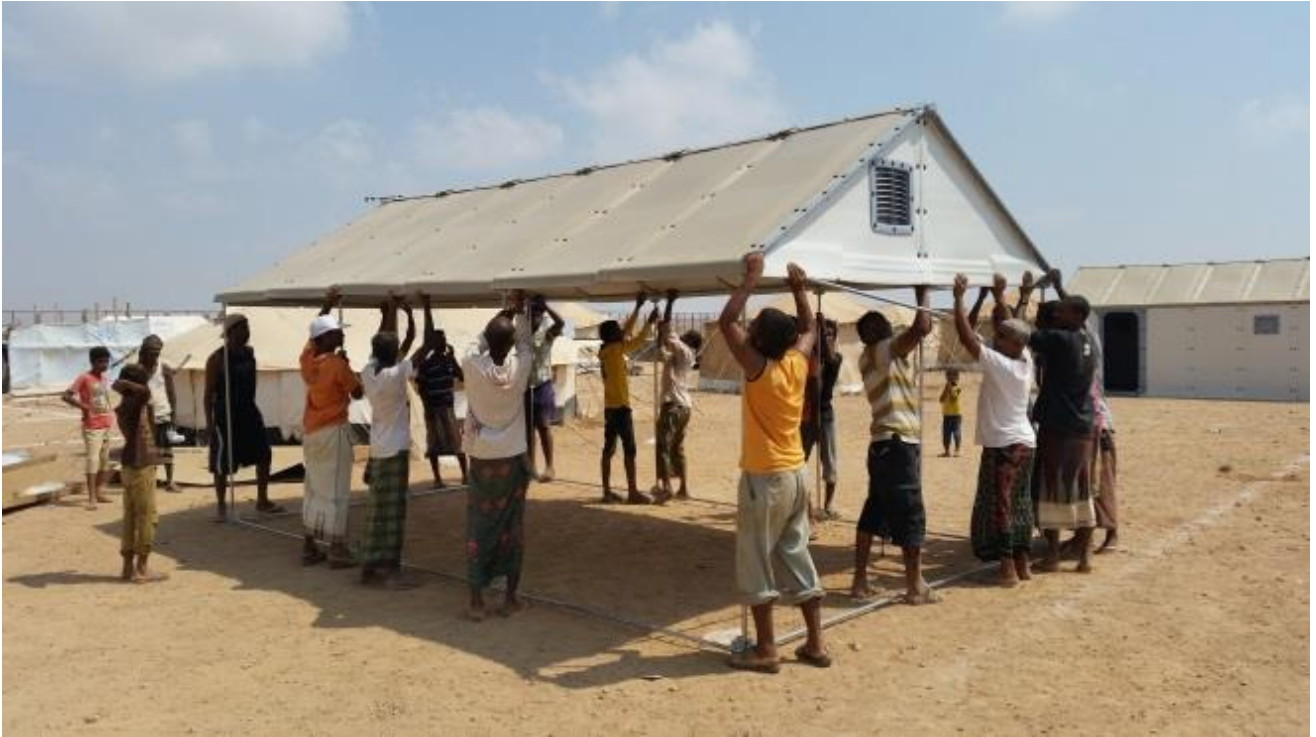
Members of the community work together to set up the Refugee Housing Units in Markazi Camp ©NRC/A. Ahmed, Oct. 2015
