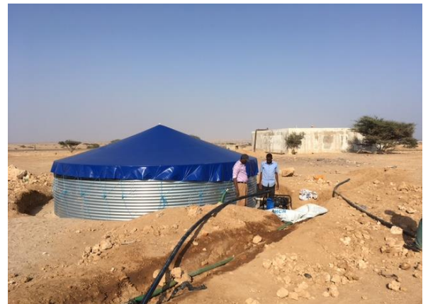
The new reservoir in Markazi camp installed by NRC and connected to the Obock main water line. @UNHCR/N.Lashermes. Feb.2017.
