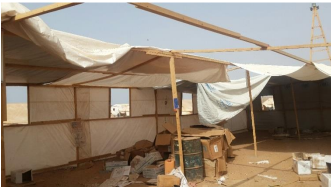
The food distribution centre has been damaged during the recent sandstorm in Obock. © UNHCR
