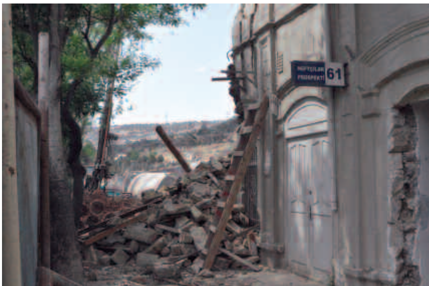
The demolished apartment building at 61 Neftçilar Avenue, in central Baku. Workers steadily demolished the building, including using heavy machinery, while residents continued to live there, and in June 2011, the last remaining residents were forcibly evicted to make way for construction of a shopping center.
