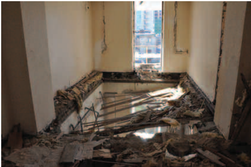
A demolished house in the area behind Heidar Aliyev Hall in central Baku. In many homes in this neighborhood and in other parts of Baku, the Azerbaijani authorities have begun to dismantle buildings while residents continued to live in them.
