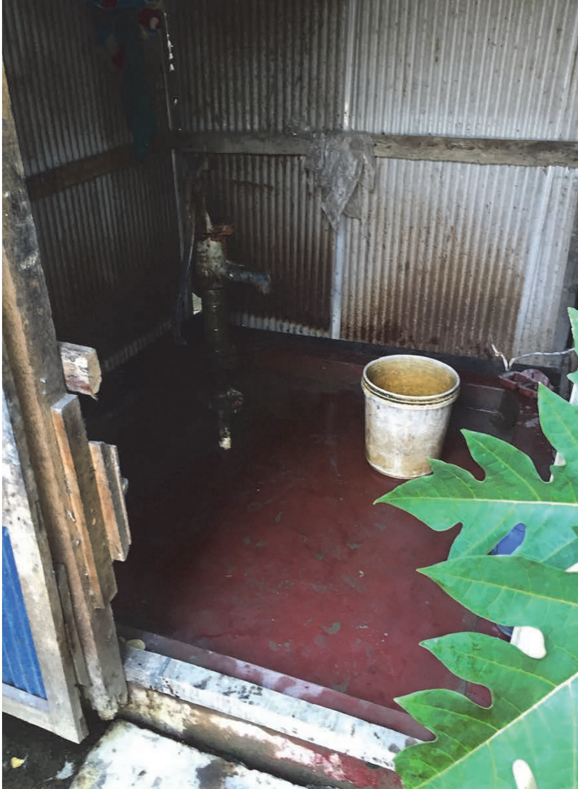
A government tubewell installed inside a small tin shed inside the fenced compound of the caretaker's house, 2015. © 2015 Richard Pearshouse/Human Rights Watch
