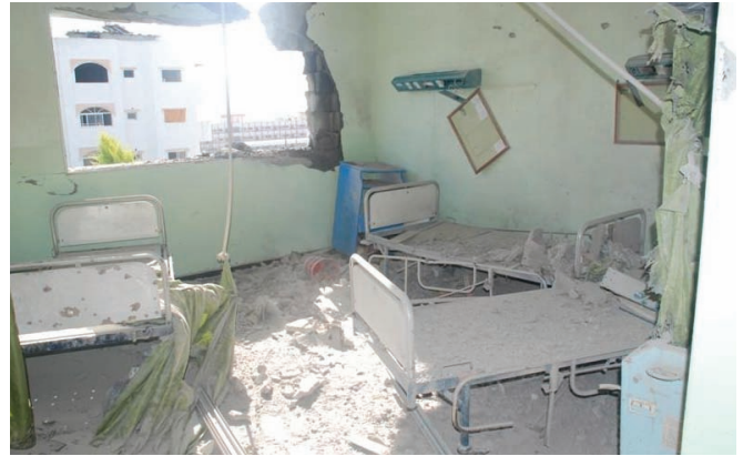
Damage within Al-Wafa Hospital
