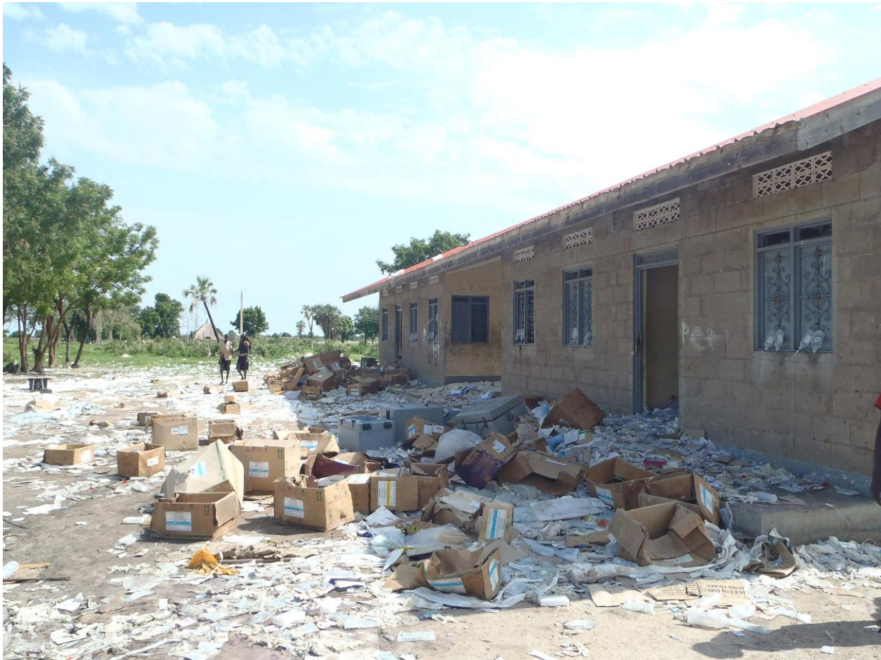
Image 2: Vandalized Koch Health Facility.
