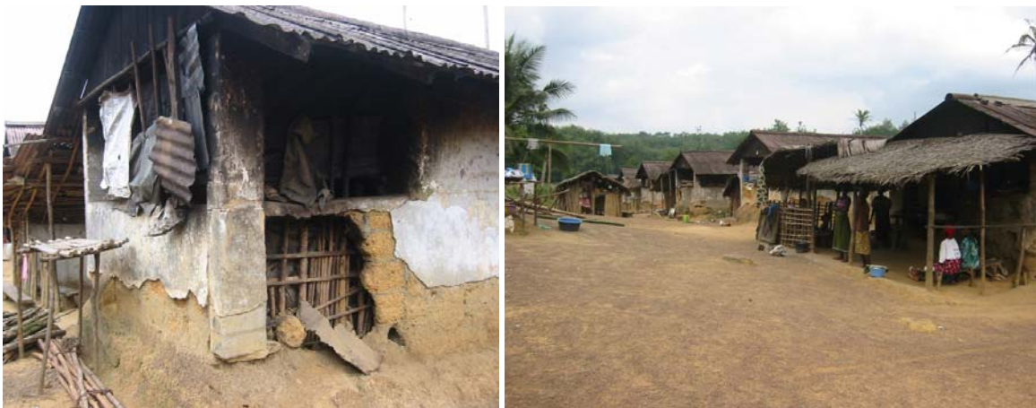
Cavalla Rubber Plantation, Camp 1, Division 3. The photos were taken by the HRO during a visit on 27 June, 2005. Workers and management stated that the houses had not been renovated since they were initially built by Firestone over 70 years ago.
