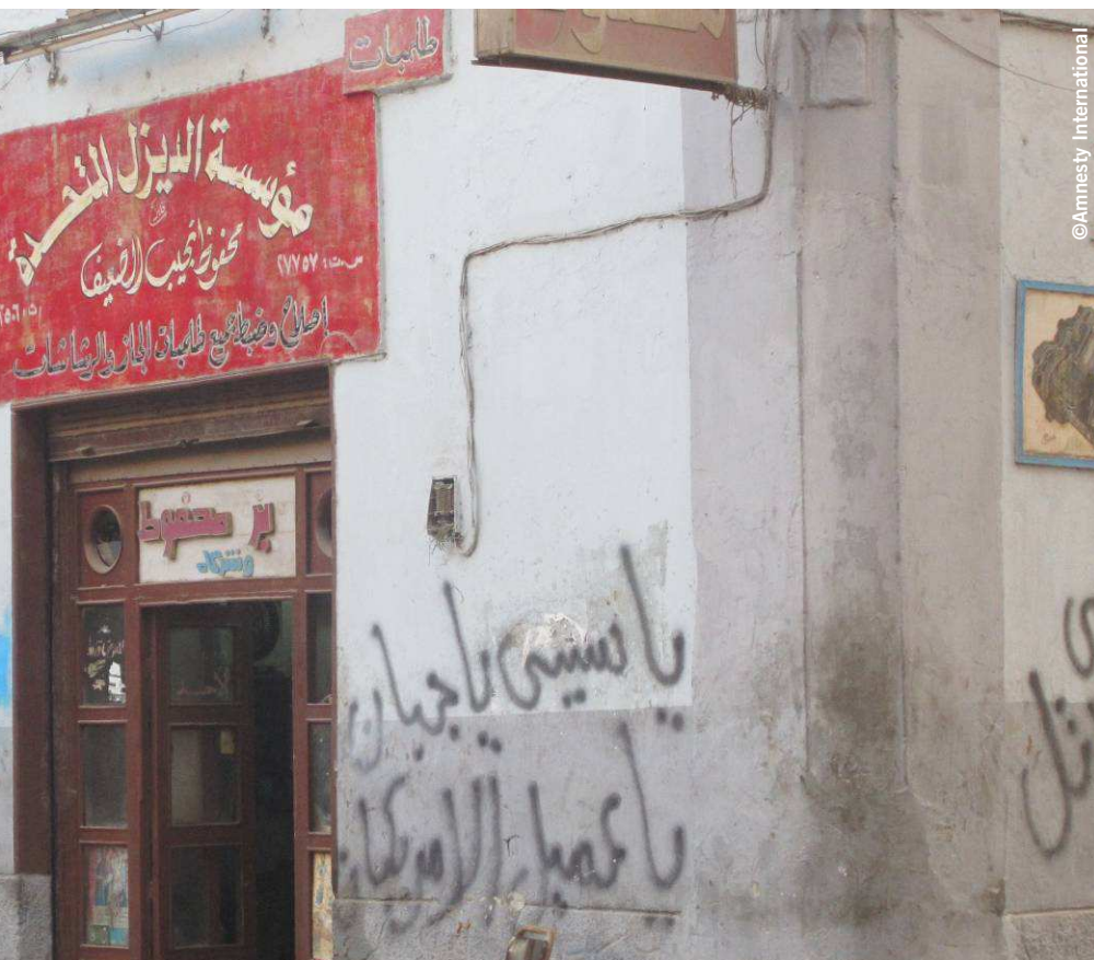
Left, overleaf: A damaged door at the Jesuit Association
