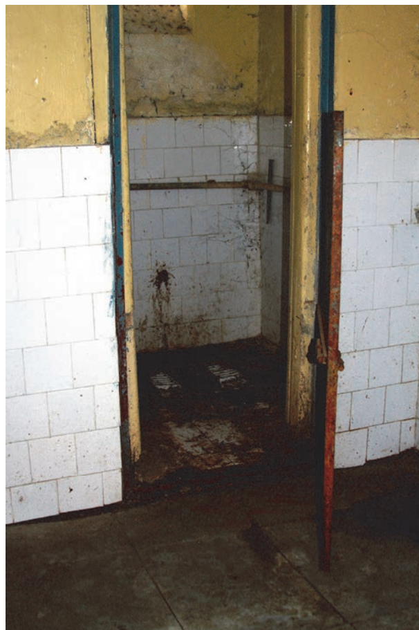
A toilet in Pune Mental Hospital, India. With only 25 working toilets for 1,850 patients, open defecation was the norm when Human Rights Watch visited in 2013 prior to renovations to its sanitation system. © 2013 Shantha Rau Barriga/Human Rights Watch
