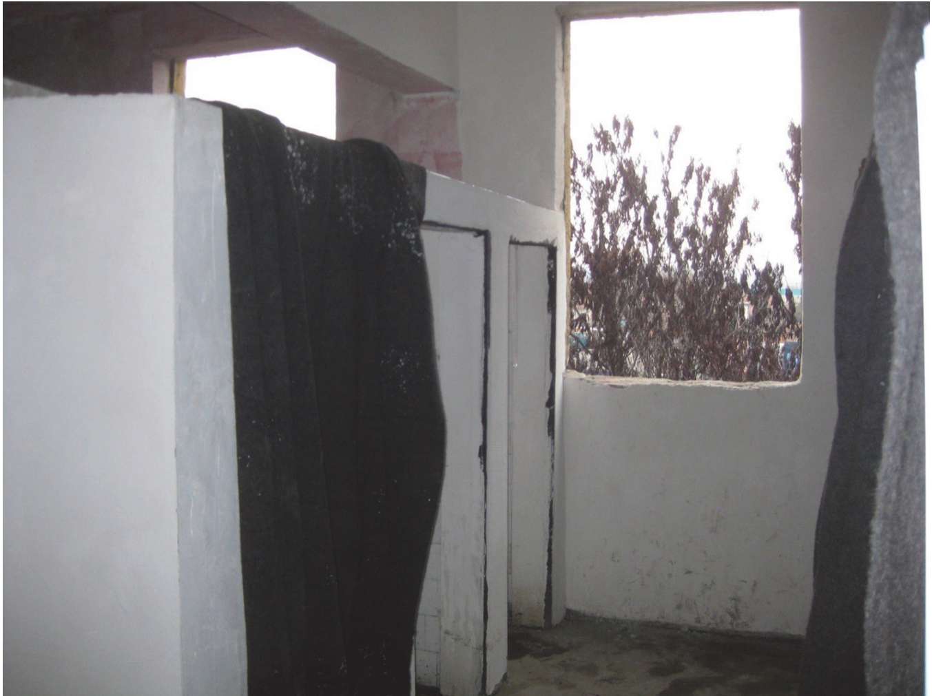
A bathroom in one of the residential buildings in the Harmanli migration center, Bulgaria. The toilets had no doors and the windows had no glass. Temperatures were below freezing. © 2014 Human Rights Watch
