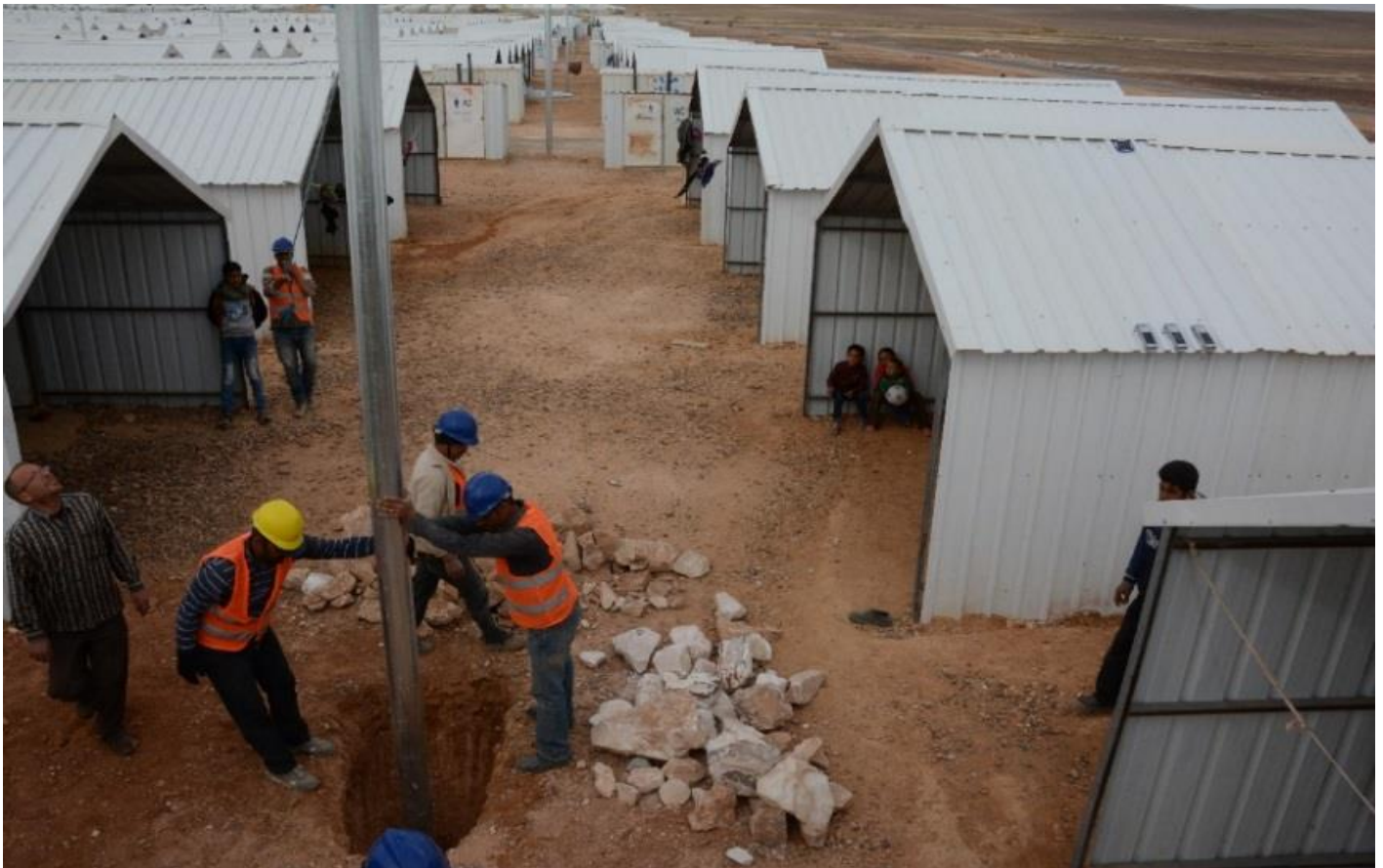
Workers installing low voltage poles as part of the first phase of an electricity project at Azraq. Improving access to a clean and sustainable source of energy can enhance self-reliance, ensure education under harsh conditions and provide safety, health and protection of refugees. ©UNHCR/A.Bino
