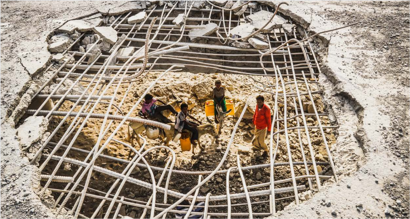
Al Hudaydah, Hajjah Road Bridge, Yemen, 2017. A man and his sons travel to collect water underneath a bridge that was hit by an airstrike in 2016. CREDIT: OCHA/Giles Clarke
