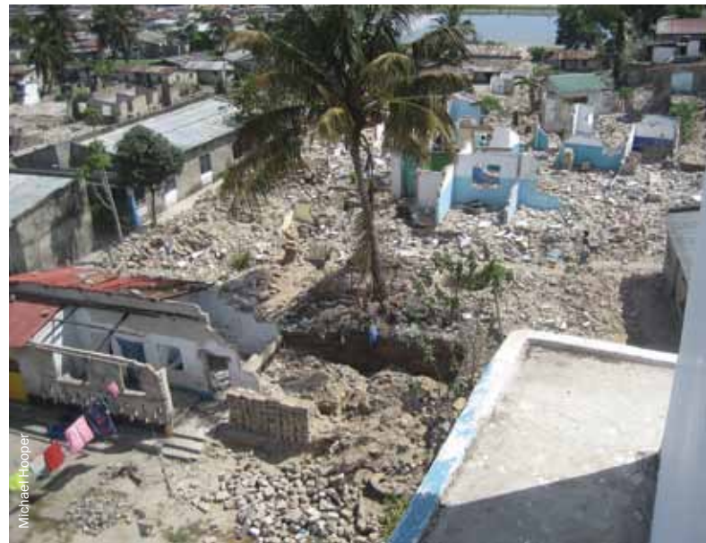
Demolished homes following evictions in Dar es Salaam's Kurasini Ward.
