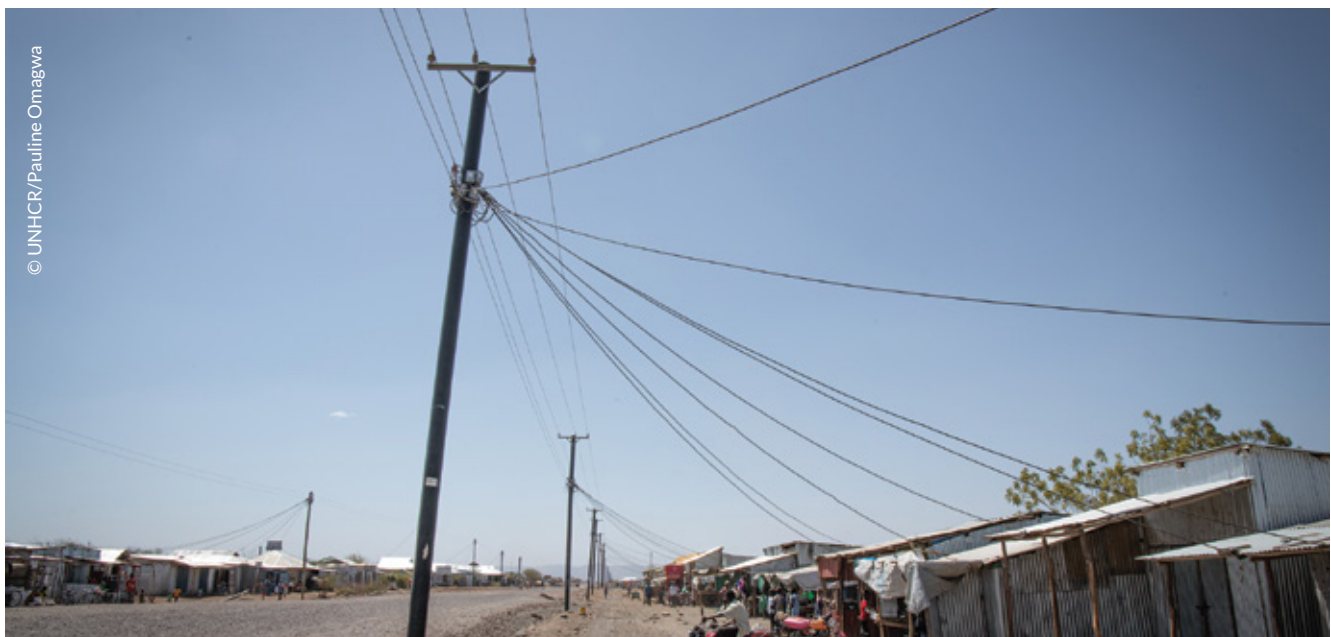
Electric poles that are part of the Kalobeyi mini grid and bring electricity to the Kalobeyi settlement.
