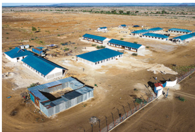
The Big Heart Foundation girls' boarding secondary school undergoing construction, set to be operationalized in 2022
