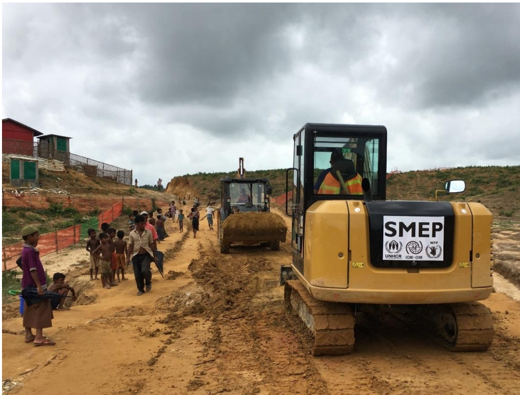
A joint UNHCR/WFP/IOM engineering project (SMEP) repairing roads in Kutupalong after heavy monsoon rains in mid-June. Photo: © UNHCR/S. O'Brien
