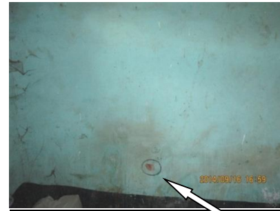
FIG 7: East side wall showing pock mark of bullet shrapnel and blood smudge on wall from which scrapings were taken
