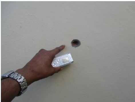
Fig 19: Bullet hole in wall of surgical theatre
