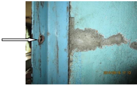
FIG 8: Door frame showing bullet mark 19 composed of a perforating defect through the metal of frame with inwardly-deflected metal edges and furrowed track across the adjacent paint/mortar or wall
