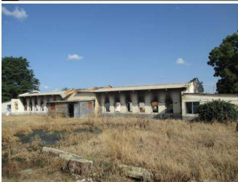
Fig 20: Paediatric ward building gutted by fire
