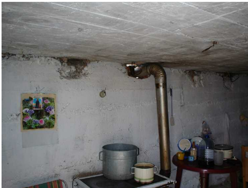
A returnee couple living in this one room of their house in the village of Cetina filed a request for reconstruction in 2001 and was still waiting for a decision in 2006. The roof leaked and the room had no heating. © CHC
