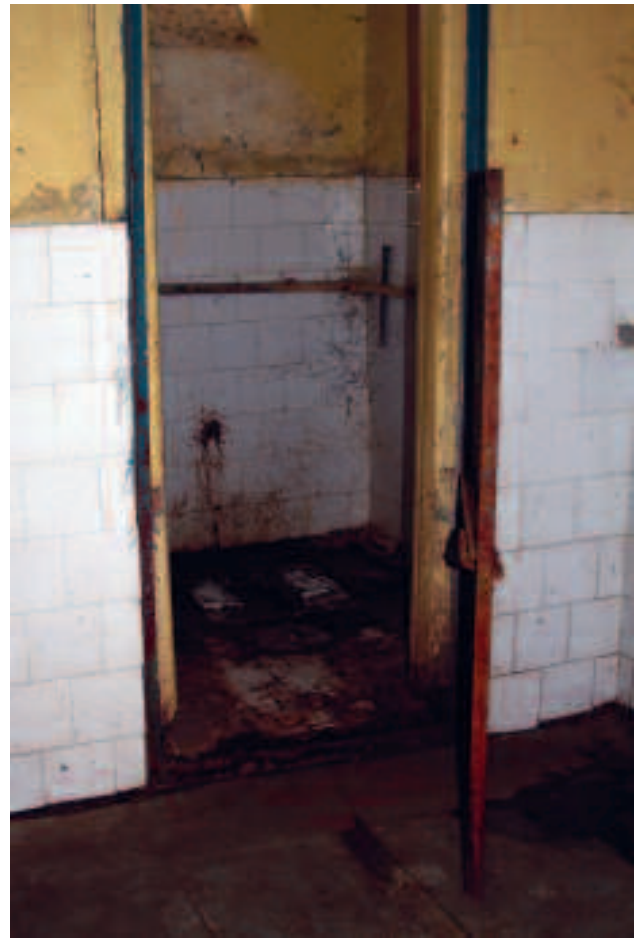
A toilet in Pune Mental Hospital. With only 25 working toilets for 1,850 patients, open defecation is the norm.
