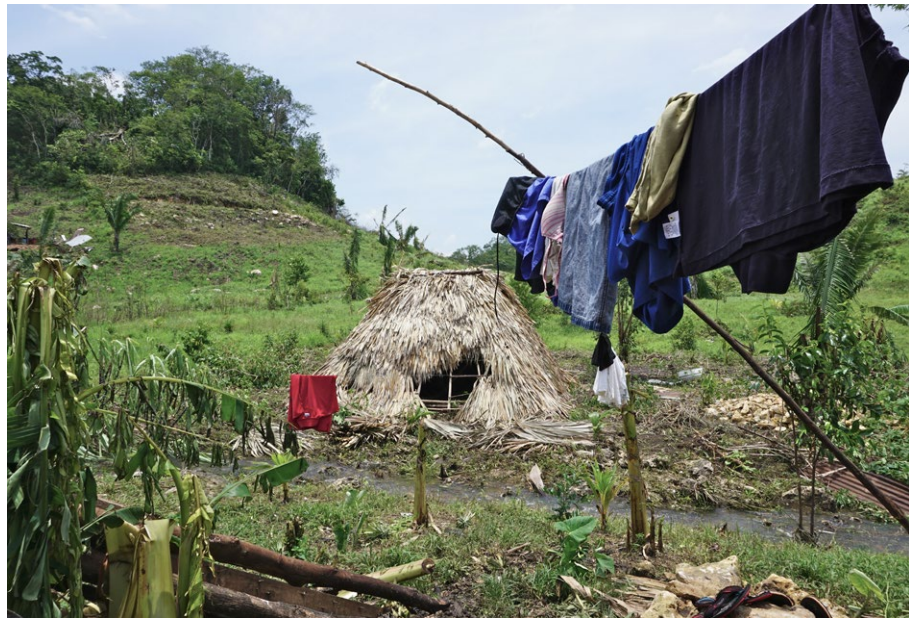
A damaged thatched-roof hut, strewn vegetation and scattered debris show the mess left behind by Hurricane Earl in a rural area of Armenia, Belize. The family that lives here are asylum-seekers, originally from Guatemala, who fled their country to seek refuge in Belize. © UNHCR/Brooke Del Greco.
