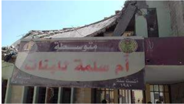
A damaged school in west Mosul
